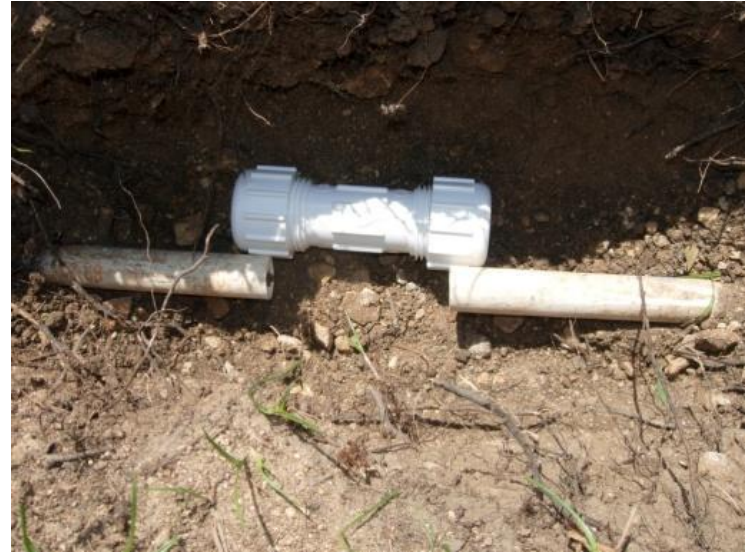
Gap is too wide for coupling
