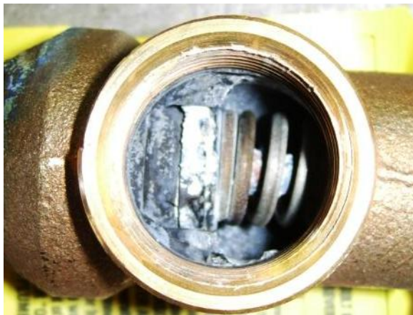
Old TPR valve has significant mineralization and corrosion around valve seat. It does not open properly; neither does it re-seal well.
