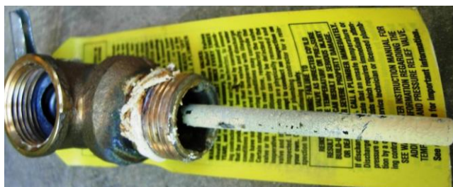
Old TPR valve has significant mineralization over temperature probe. It may open at a higher temperature.
