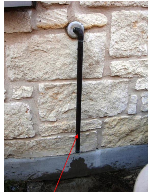
Safety valve discharge pipe (drain)
