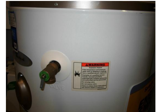
TPR Valve on Side
