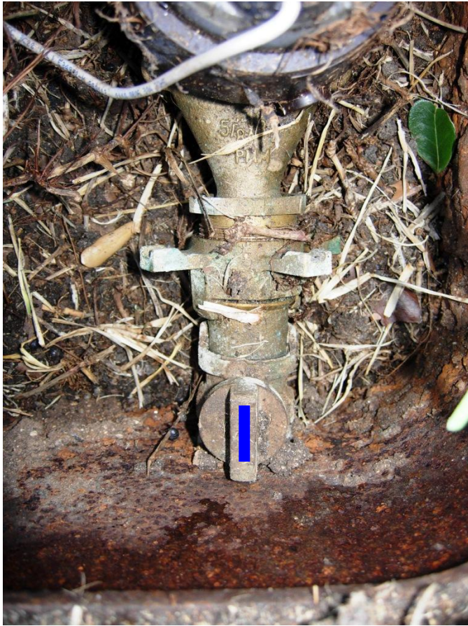
Valve Open (Water On )
