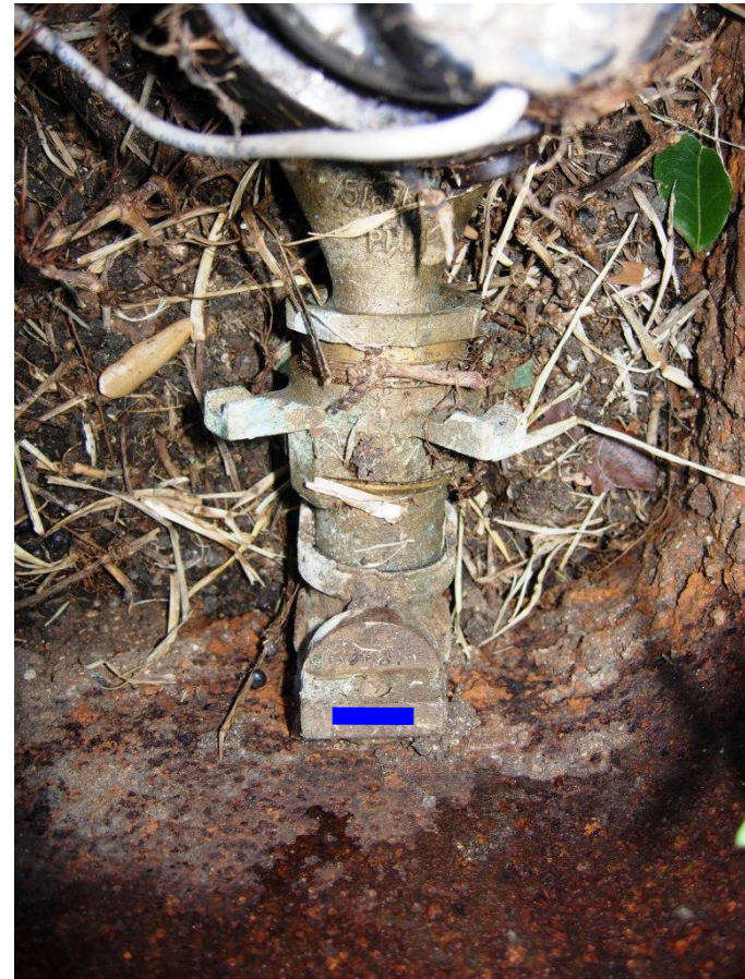
Valve Closed (Water Off )
