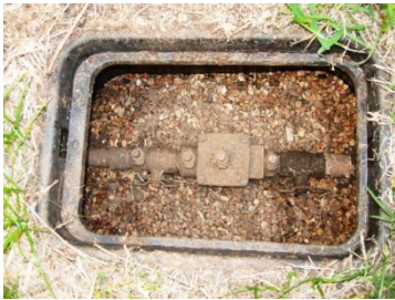
Double Check Valve (Backflow Preventer)
