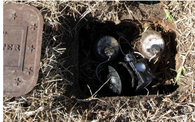
Typical In-Ground Water Meter
