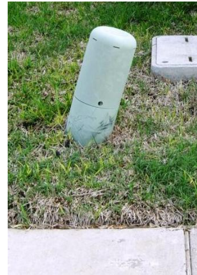
Cable Pedestal Can be Straightened
