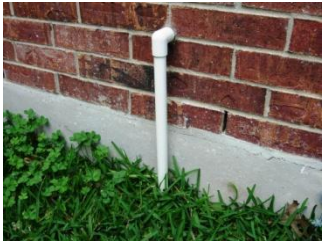
Valve Wires in Conduit From Controller
