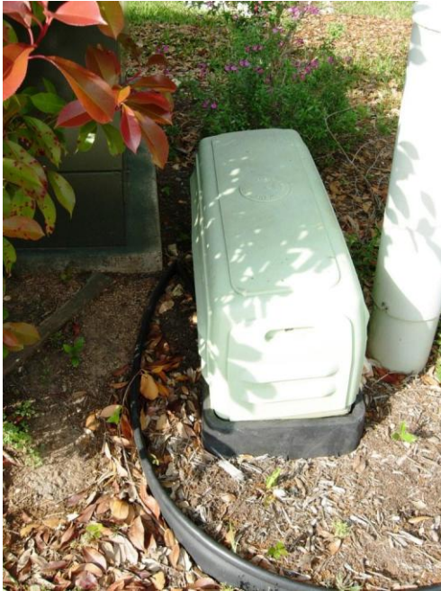
Cable Distribution Box
