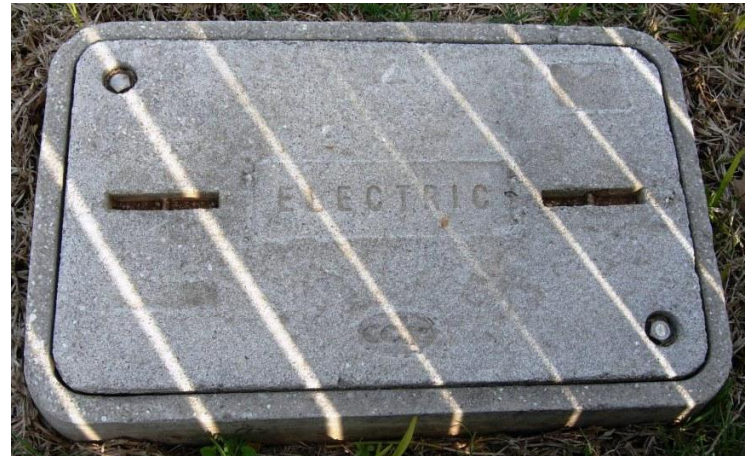
Typical Service Box
