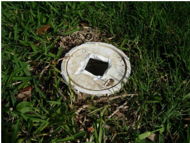
Broken Cleanout Cover
