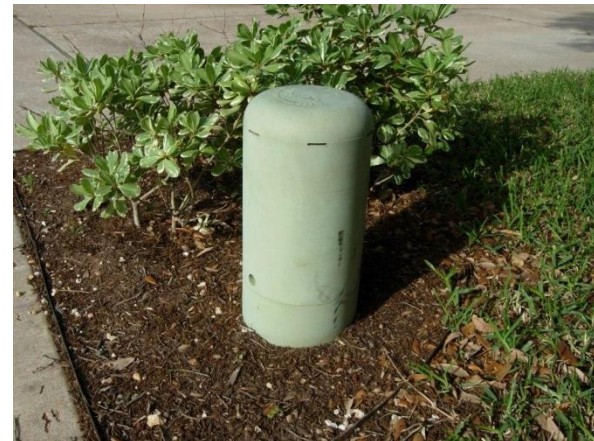
Cable Distribution Pedestal
